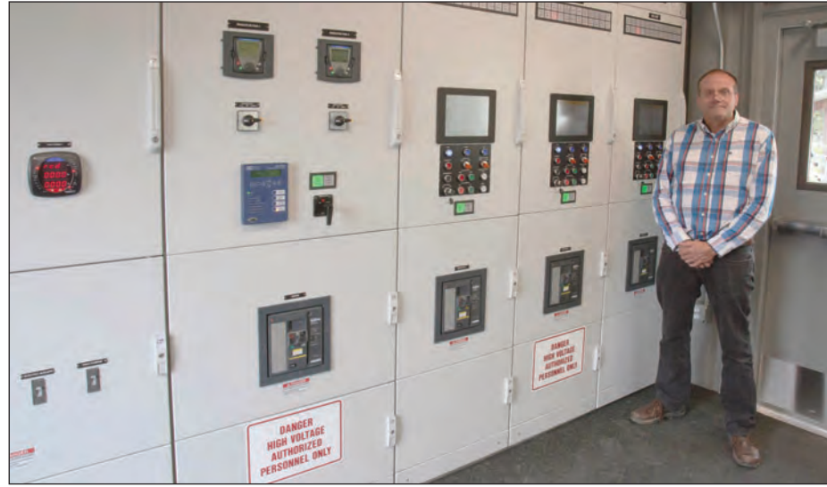
Alaska Energy Authority project manager Alan Fetters in the control room of the new powerhouse for the village of Perryville. The state-of-the-art control system integrates the powerhouse's diesel generators with Perryville's wind farm and power grid, provides continuous monitoring of the power supply system and remote access for offsite monitoring and assistance.
